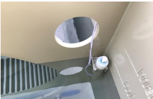
Float is in 'normal' position, pond pump is on
